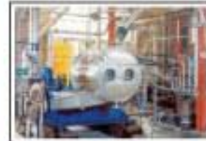
INDUSTRIAL PROCESSING TECHNOLOGY
